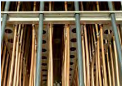
Internal view - cooling pipes
