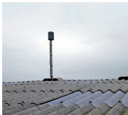
Roof mounted antenna
