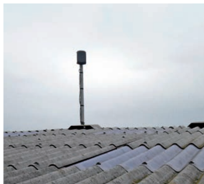
Roof mounted antenna
